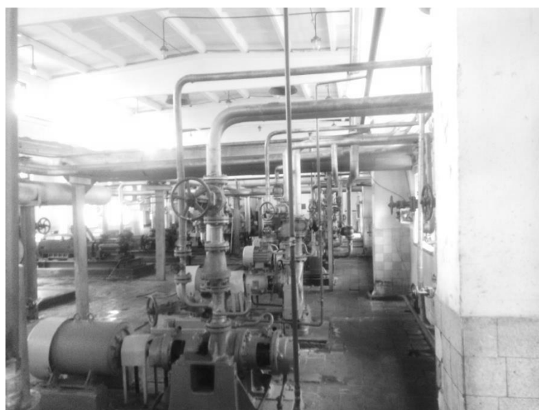
Fig. 5.12. General view of the location of centrifugal pumps at the Dolinsky GPP
