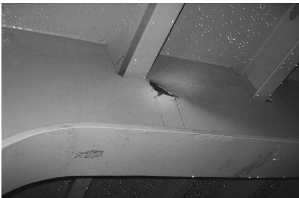
Fig. 2. Deformations of the floating dock body: a) significant bending of the tower and pontoon; b) metal deformation under the slipway-deck
