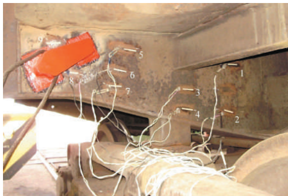
Figure 5.13 – Location of strain gages on the vertical sheet of a car bolster beam
