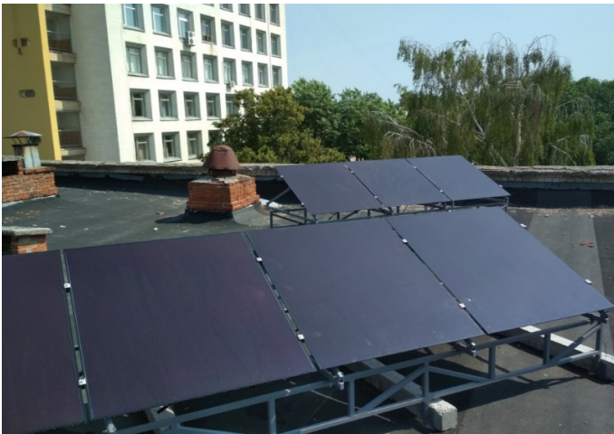
Fig. 4.1. Photovoltaic power station at Chernihiv Polytechnic National University
