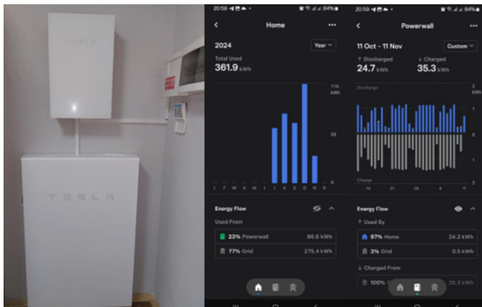
Fig. 4.2. External view of the Tesla power wall system and information application
