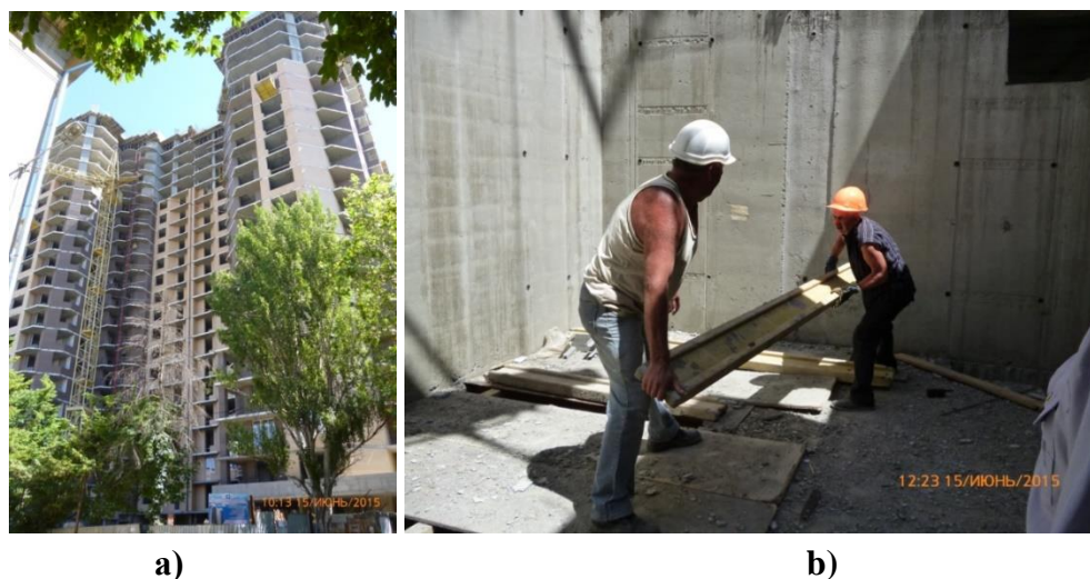
Figure 10. Object of field studies, a) – Photo fixation of facility b) – Tamper strikes in the elevator section
