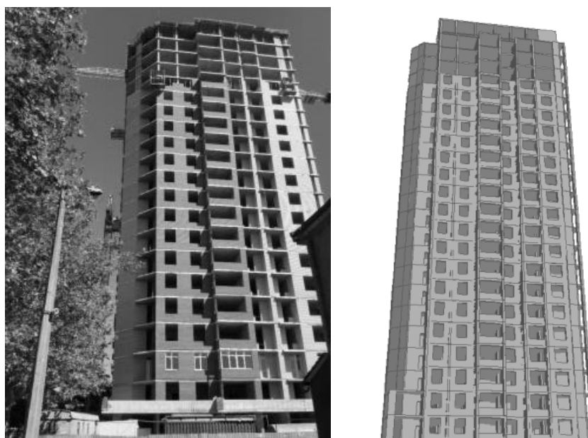
Fig. 11. General view of the tested building and design scheme with regard to the wall fencing
