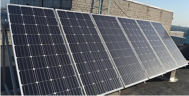
Fig. 4. General view of the section of photovoltaic modules mounted on the roof, TS
